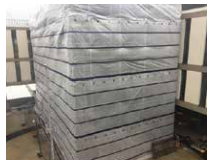
"Birdcage" Renovation: Work begins on the signature staircase affectionately known as the birdcage. The $800,000 project is funded by Milwaukee County.
