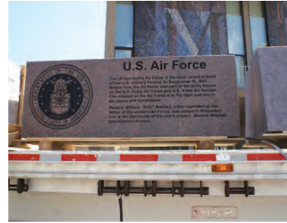
Granite Bollards: The new markers installed in front of WMC protect the building against traffic and honor our military history.
