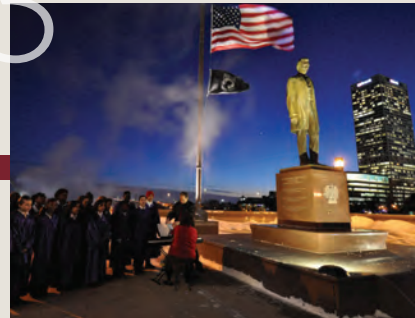
Fall 2013: Restoration to the west facade Lewandowski Mosaic Mural & lighting of the Lincoln Statue.
